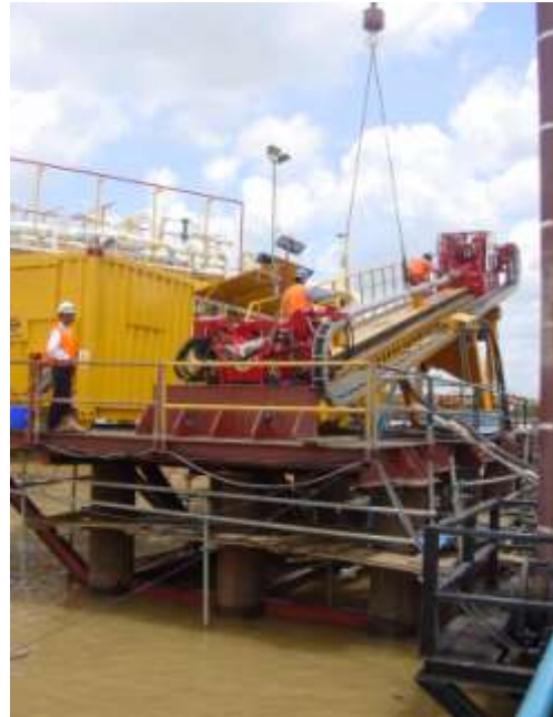
Picture 6b Drilling from offshore: Pipeline construction with a Herrenknecht HDD rig in Indonesia
