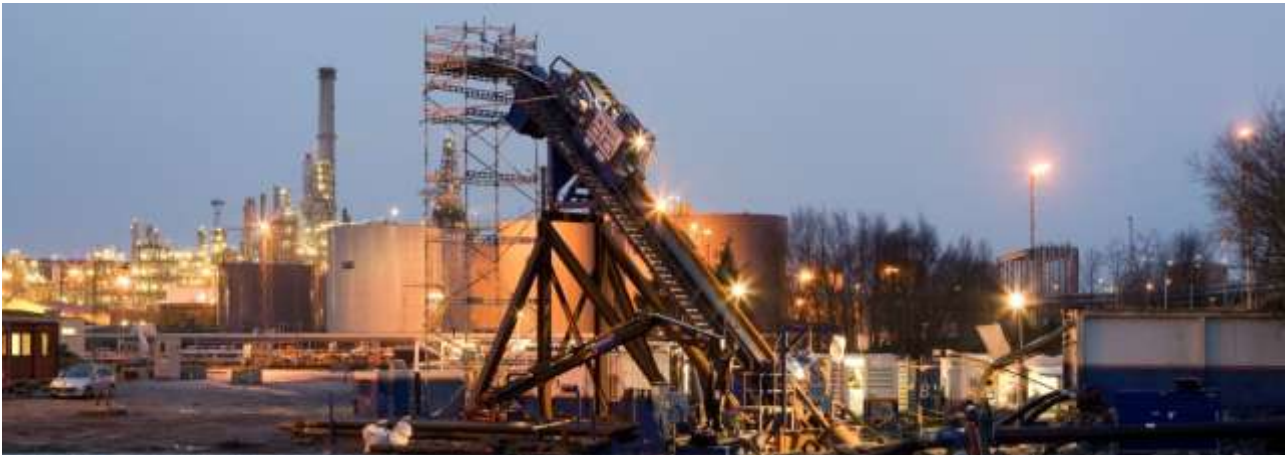
Picture 4: Drilling starting onshore: The Herrenknecht HDD HK250T machine in Norway, rock drillings for a landfall tunnel – 20” gas pipeline with gradient
